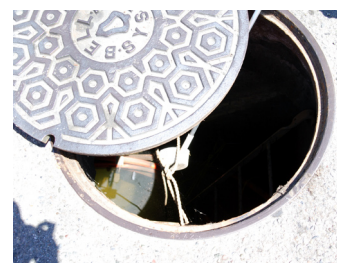
An underground vault full of water and mosquitoes
