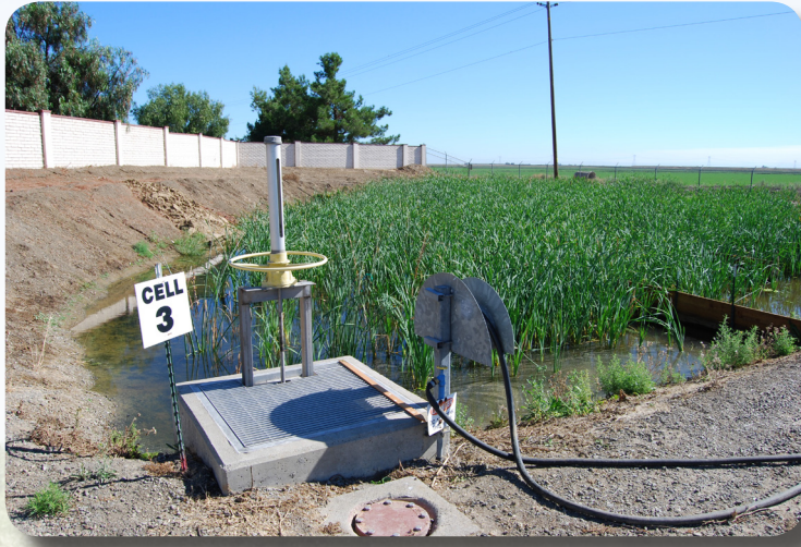
Discovery Bay Wastewater Treatment Plant
