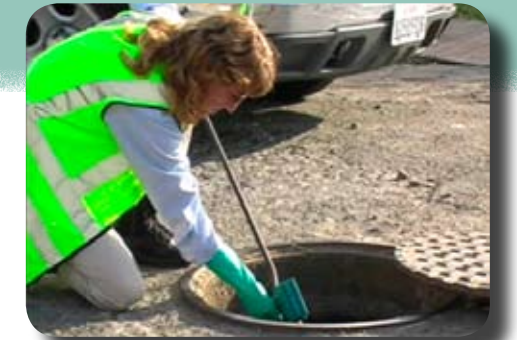
Fig. 2 Vector Control Inspector Nancy Harden places bait for rats in city sewers
