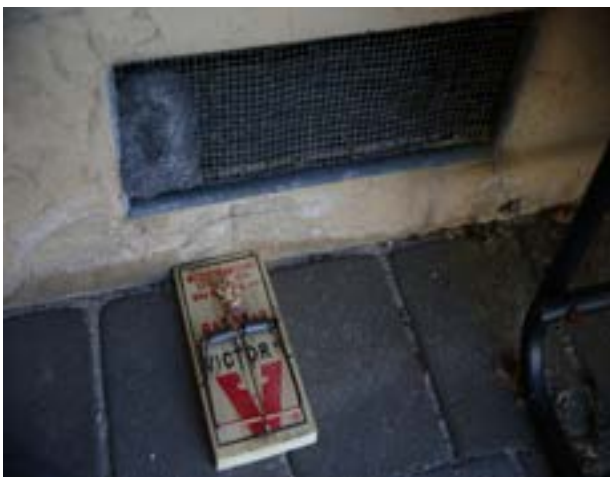
A damaged vent screen can be an entry point into a home for mice.
