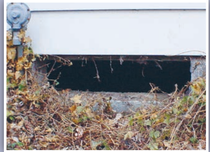
Damaged or missing vent screen provides skunks access under a home**
